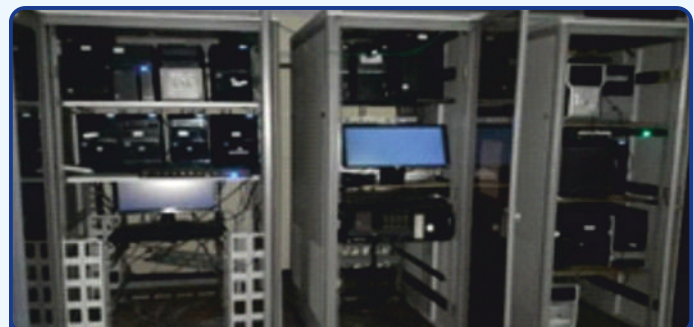
Centralized Server systems
