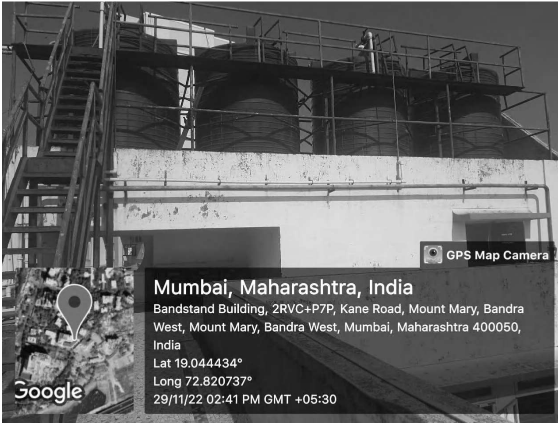
Four Water tanks with 15000 lits. capacity
