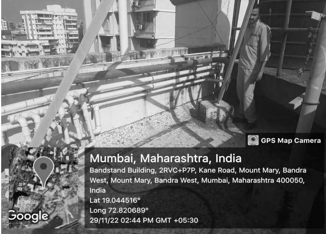
Outlet pipes for rain water harvesting
